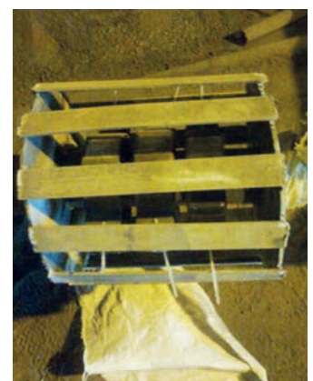
Fig 5. Magnetic water conditioners on balling plant water lines
