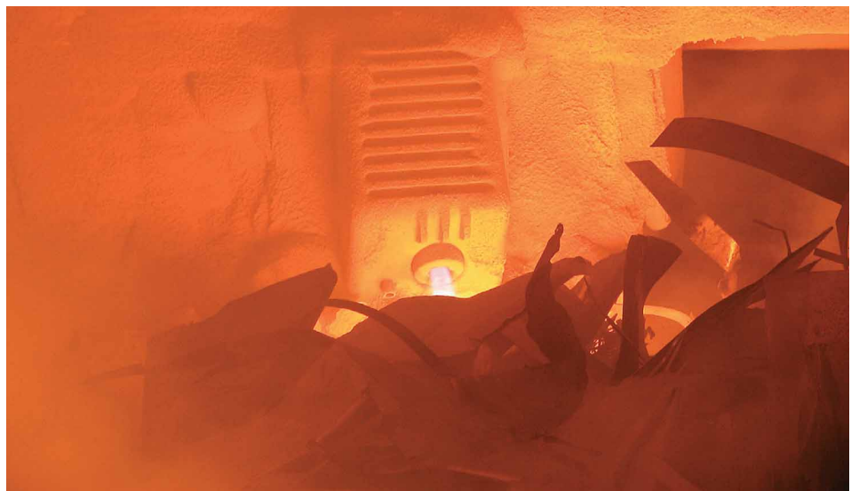
JetBOx™ is mounted on the sidewall close to the metal loath
