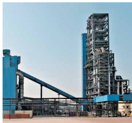
Fig 4 Inclined hot transport conveyor at Hadeed Module E
